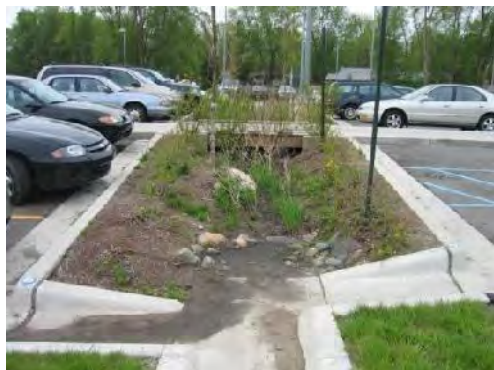
The bioretention area in this parking lot island has accumulated sediment which requires removal.
