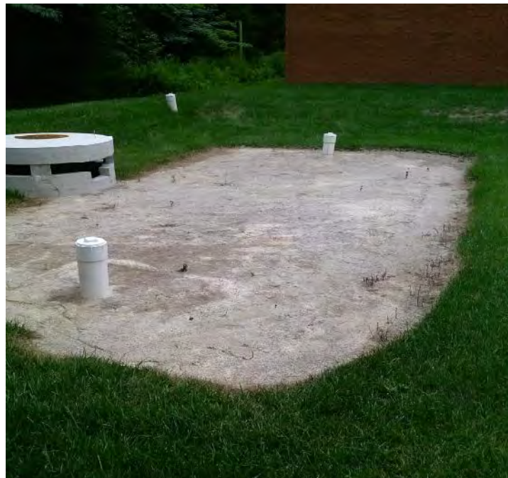
Observation wells in infiltration area
