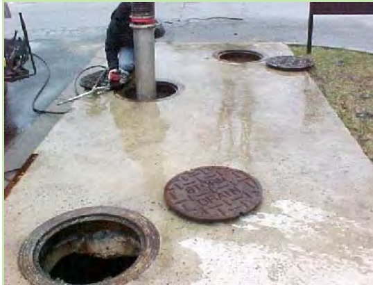
Figure 6.20.1: Maintenance of a Manufactured Treatment Device
