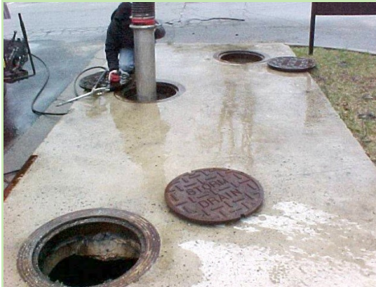
Figure 6.20.1: Maintenance of a Manufactured Treatment Device
