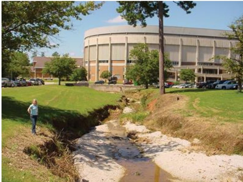
Figure 1-6. Parkerson Mill Creek Erosion, Auburn AL (Source: Storm Water Solutions Newsletter, Feb. 6, 2017)
