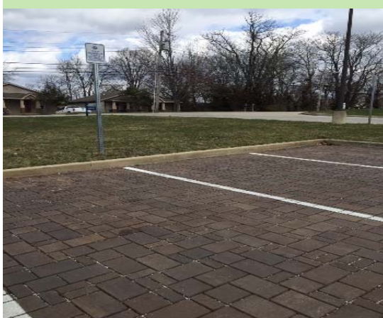
Above: Permeable pavers reduce the impervious surface of parking lots and provide a multi-functional value to the developer.
