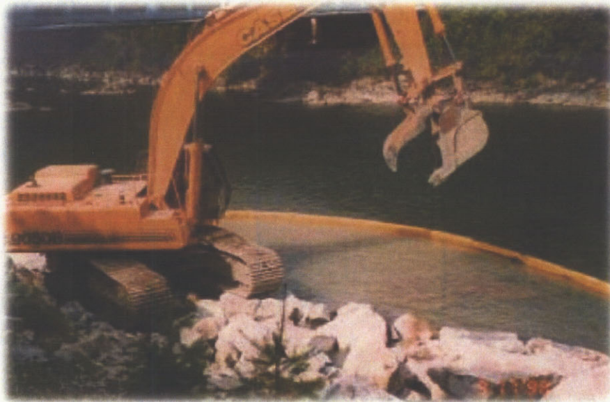
A turbidity curtain being used to contain turbid waters during construction activities
