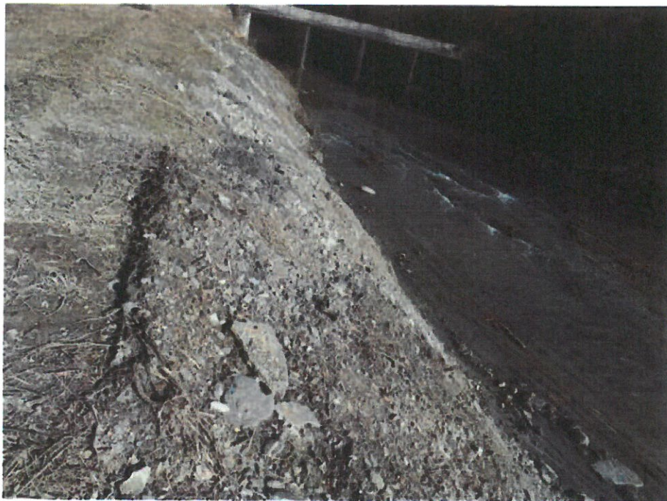
Disturbed Creek Banks
